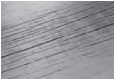
Weathered wood structure *
